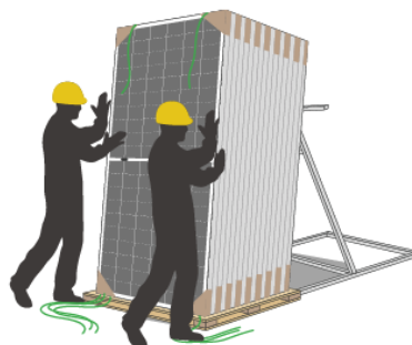
8) Cut off the remaining packing belts so that the modules rest on the stand supporter.
